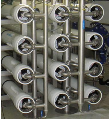
Reverse osmosis skid
